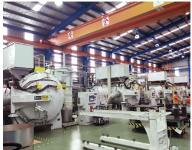
中壢一廠硬焊設備 Brazing facility in Chung-Li Plant 1
